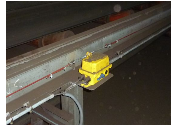
LHPE conveyor stop switch
