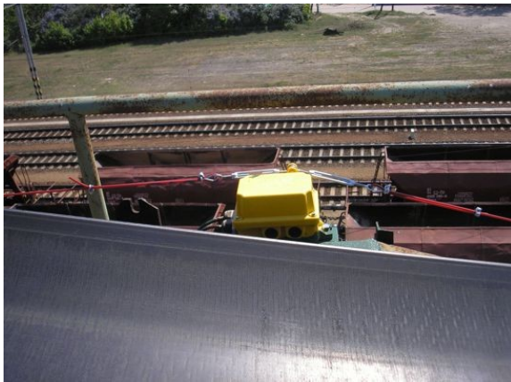
LHPE conveyor stop switch
